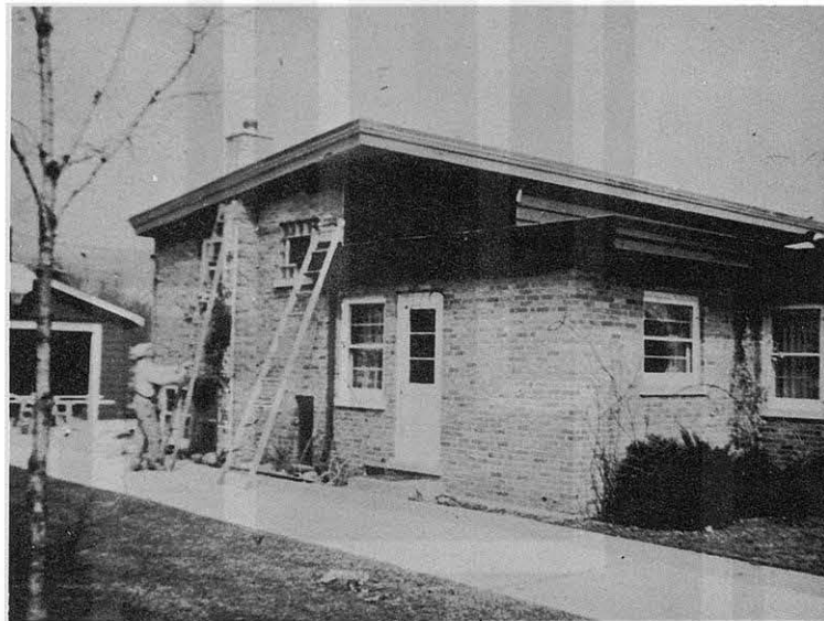
Fig. 12 One of the two houses on Evergreen Road that had its roof blown off. (Picture taken during placement of new roof.)
